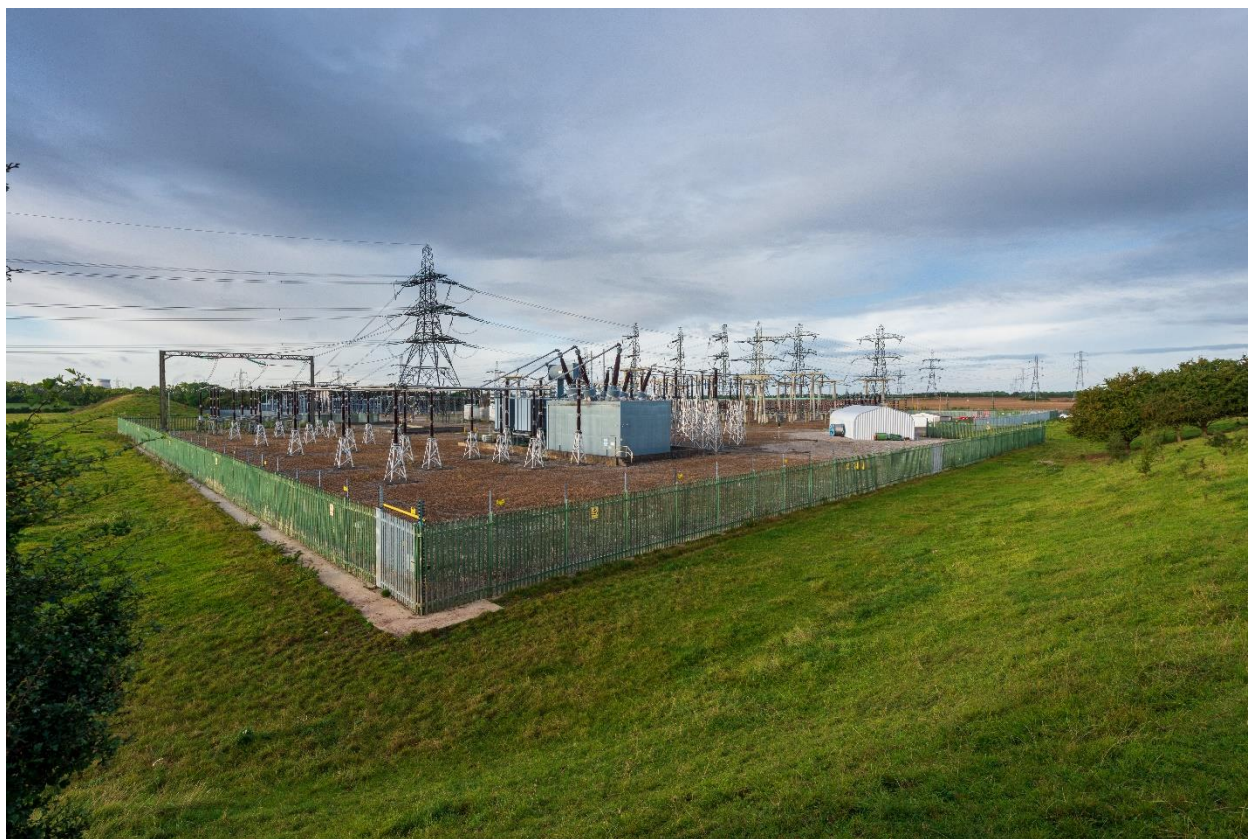
Figure 2.3 – Typical substation (existing Monk Fryston Substation)
